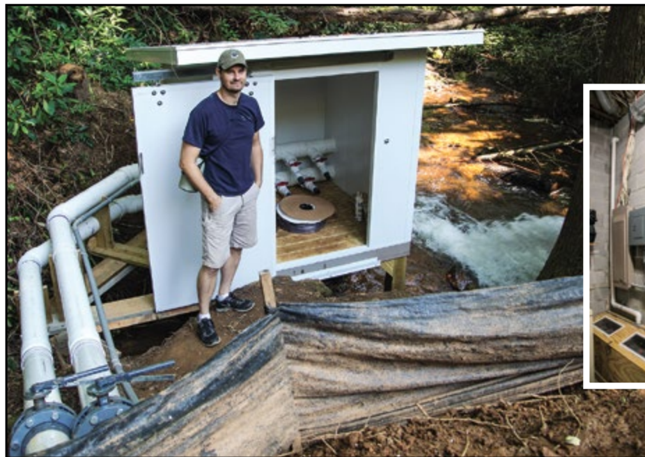
Above Lft: S-Tek Building Solutions COO, Jason Smith in front of completed Penstock Outtake & Generator House (river side). Above Rt: Inverter battery box, diversion controller, diversion loads & essential inverter load panel.
