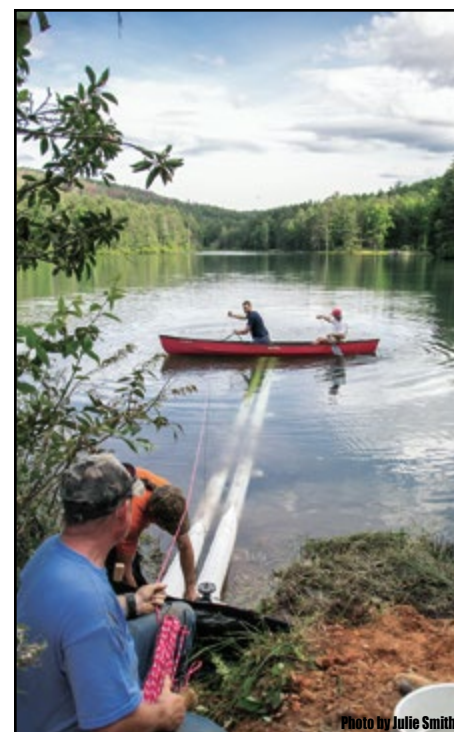
S-Tek Building Solutions Crew and homeowner Don George installing the Intake Piping at the main water source (lake side).
