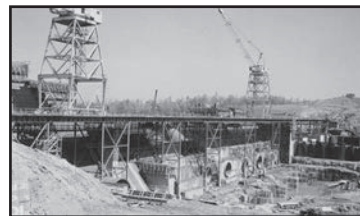
Above: The Lake Hartwell dam under construction in 1959 (photo courtesy U.S. Army Corps of Engineers)
